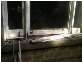
Decayed timber frame and cill
