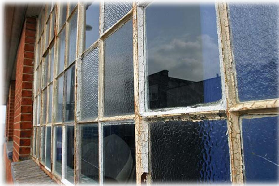
Fig. 3 Metal window demonstrating lack of maintenance
